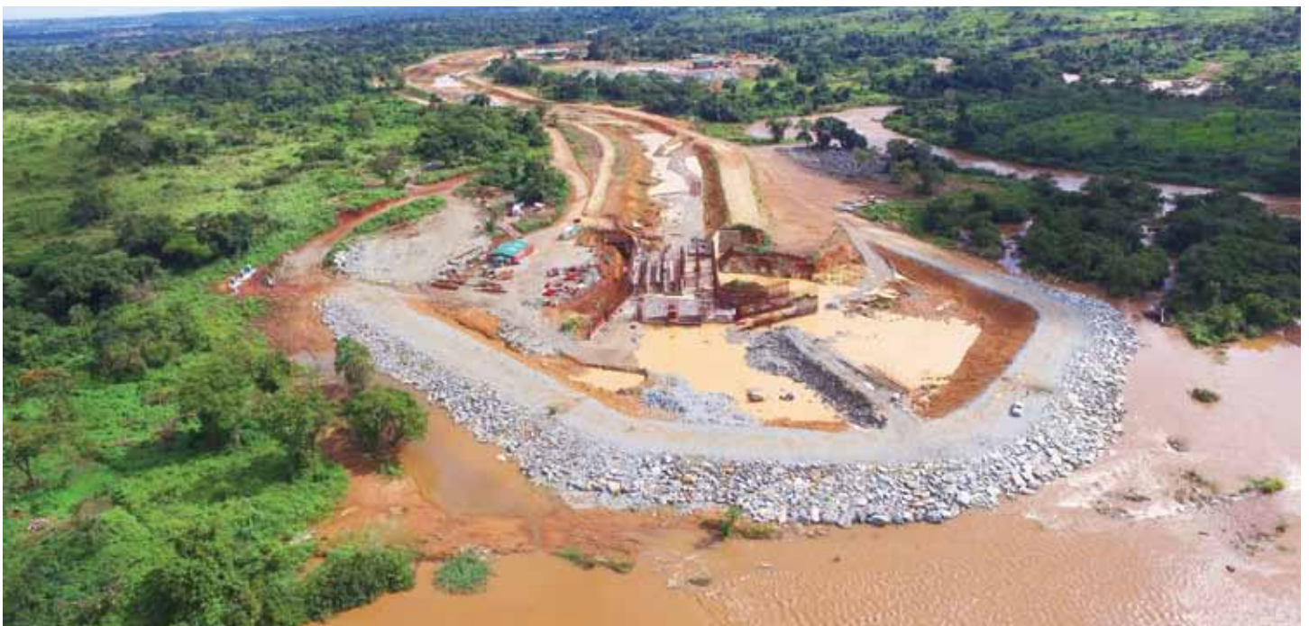
View from the intake system. The all-Congolese contracting team is making good progress with the construction of Kibali's third new hydropower station, Azambi.
