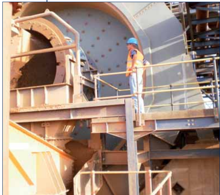
Chief engineer Awie Frey oversees commissioning of the first mill at Tongon.
