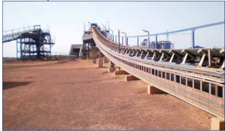
First ore on the conveyor to the newly commissioned metallurgical plant.
